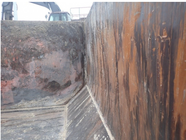
(Photo 5) Overview Of Distortion 2
