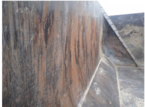
(Photo 4) Overview Of Distortion
